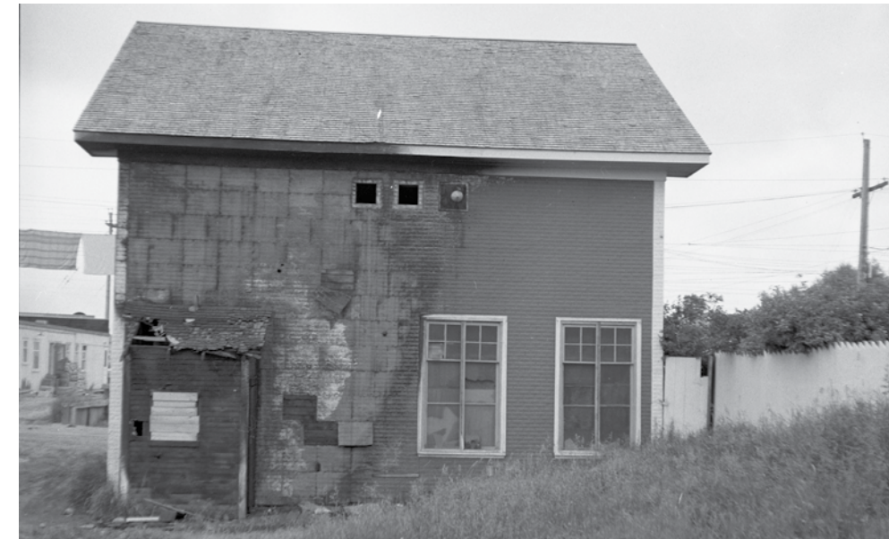
The former City-owned powerhouse at 1515–34 Avenue SW functioned as a Scout Hall from about 1939 until at least 1961. This 1955 photograph shows fire damage caused by arson.
